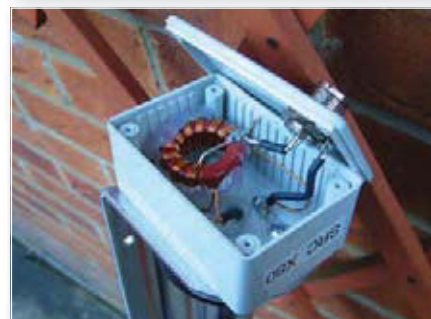
Fig. 12: The 9:1 ratio UnUn transformer on the X80 antenna.
